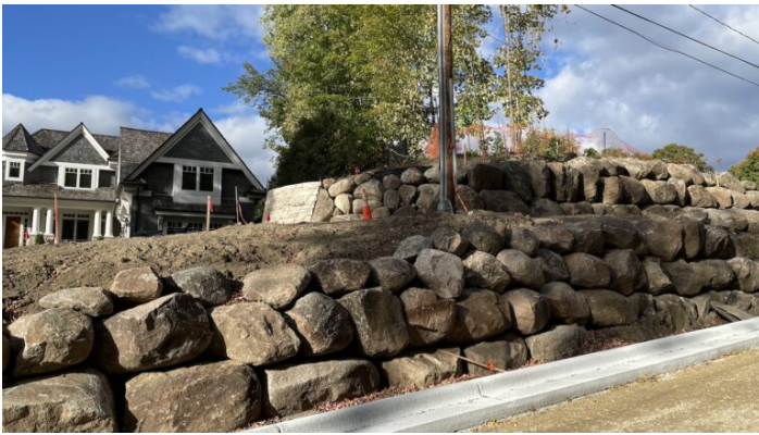
Huge construction project on Birch Bluff Road, just around the corner from the Blomquists
