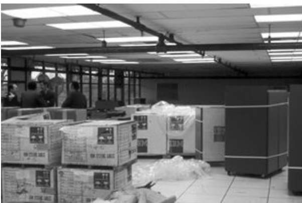
Installation of the SLAC Triplex
